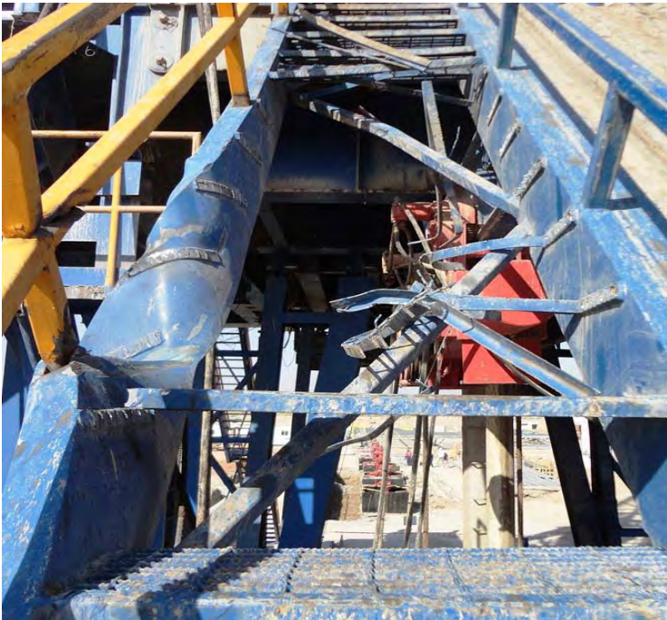
Catwalk Stairs damaged by flying fragment of Pulsation Dampener
